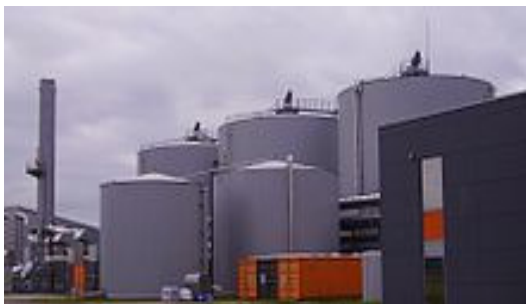
Anaerobic digestion component of biological treatment plant
